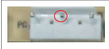
Measure the voltage of this foot to neutral wire on the mainboard
